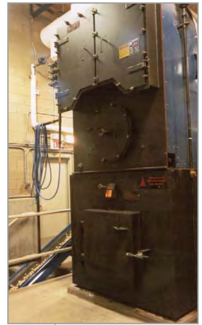
Opposite page: The woodchip-fired biomass heating plant at the Darby school system.
