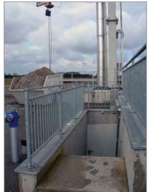
Opposite page: Aigner Engineering’s below-ground biomass plant on the premises of the Fronius manufacturing plant in Upper Austria.
