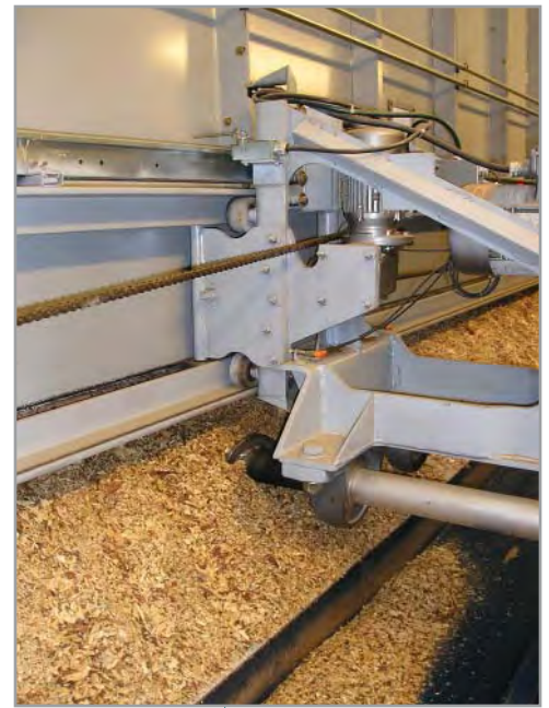
Opposite page: STAR Academy’s three-bay chip storage facility.
