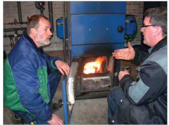
Opposite page: This small pellet boiler plant heats all the buildings of the Zoo School.
