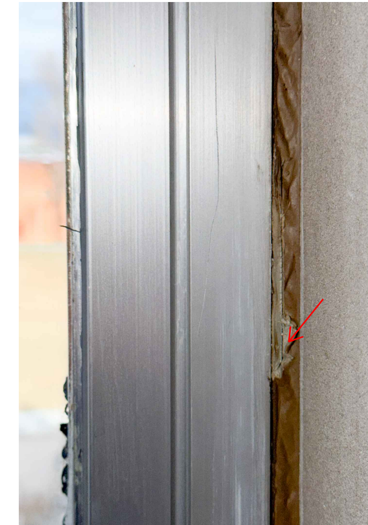
PHOTO 1: EXAMPLE IMAGE OF UNPAINTED M2.1 (TAN CAULK) ALONG WINDOW CASING. ABATEMENT REQUIRED AS DISCUSSED IN DETAILS 1 AND 2 (SECOND FLOOR) AND DETAILS 3 AND 4 (THIRD FLOOR).
