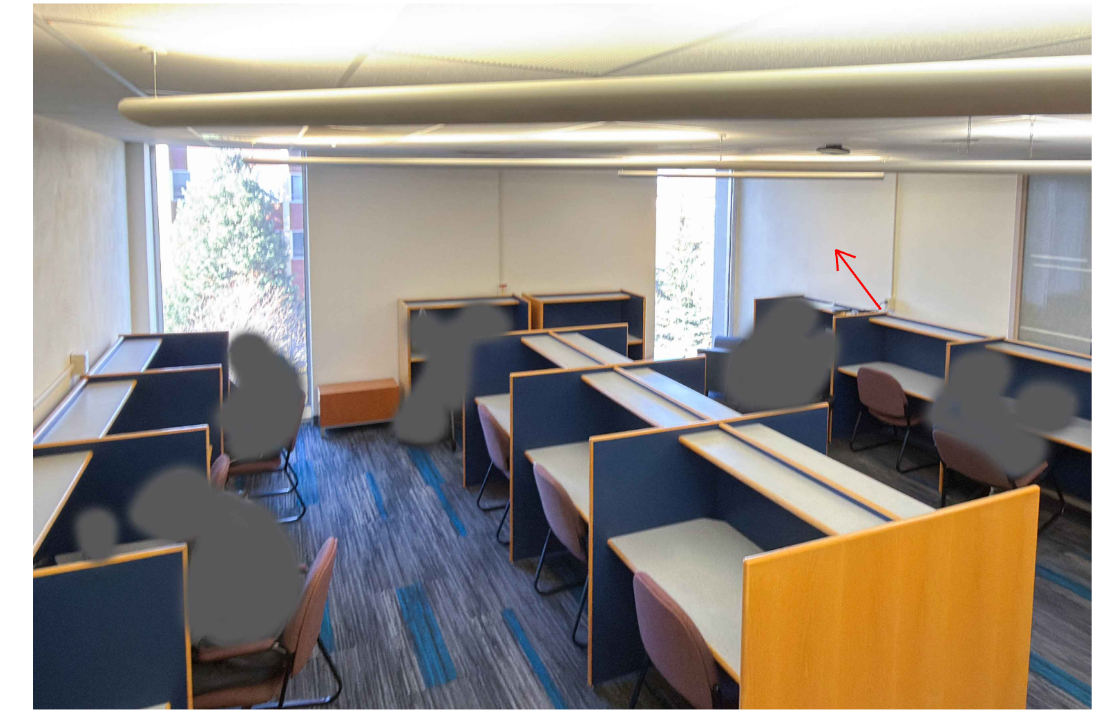
PHOTO 2: EXAMPLE IMAGE OF P1.1 (PLASTER WALL) ADJACENT TO WINDOWS ALONG WEST SIDE. AVOID IMPACTS AS DISCUSSED IN DETAIL 2 (SECOND FLOOR) AND DETAIL 4 (THIRD FLOOR).
