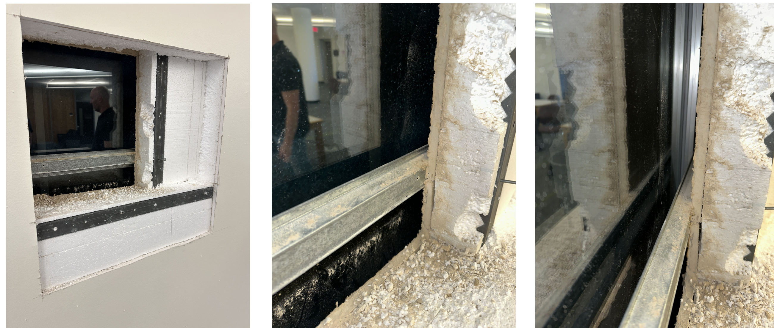
INVESTIGATION HOLE AT WALLS IN FRONT OF EXISTING WINDOWS TO SHOW EXTENT OF WALL CONSTRUCTION.
