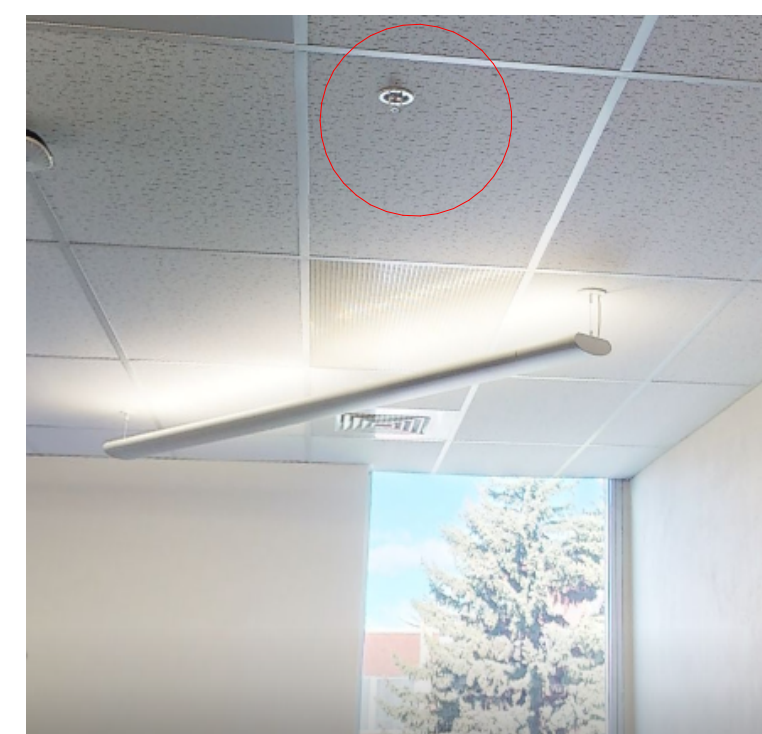
PHOTO OF EXISTING PENDANT SPRINKLER ALONG WEST WINDOWS TO REMAIN. 13'-6" FROM GRID LINE 1.
