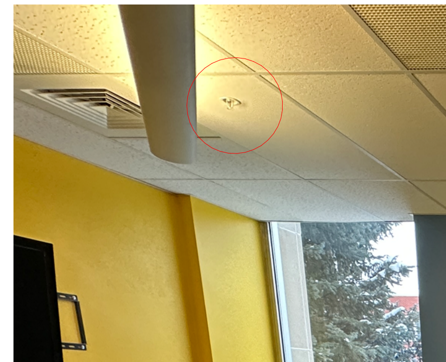
PHOTO OF EXISTING PENDANT SPRINKLER ALONG WEST WINDOWS TO REMAIN. FIRST ROW IS 5'-5" FROM GRID LINE 1, SECOND ROW IS 13'-3" FROM GRID LINE 1.
