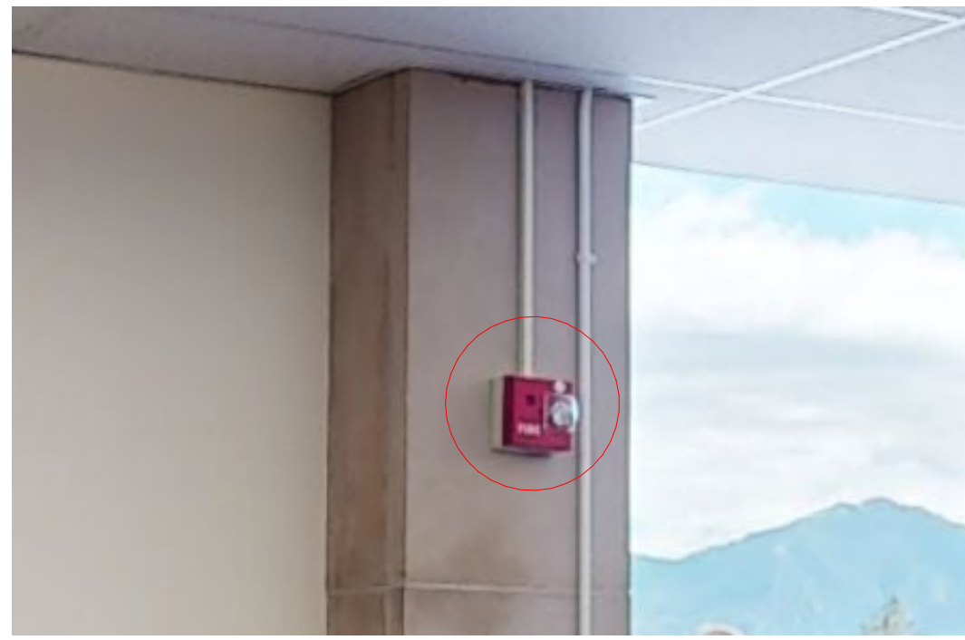
PHOTO OF EXISTING FIRE DEVICE LOCATED AT GRID LINE 4-A TO REMAIN.
