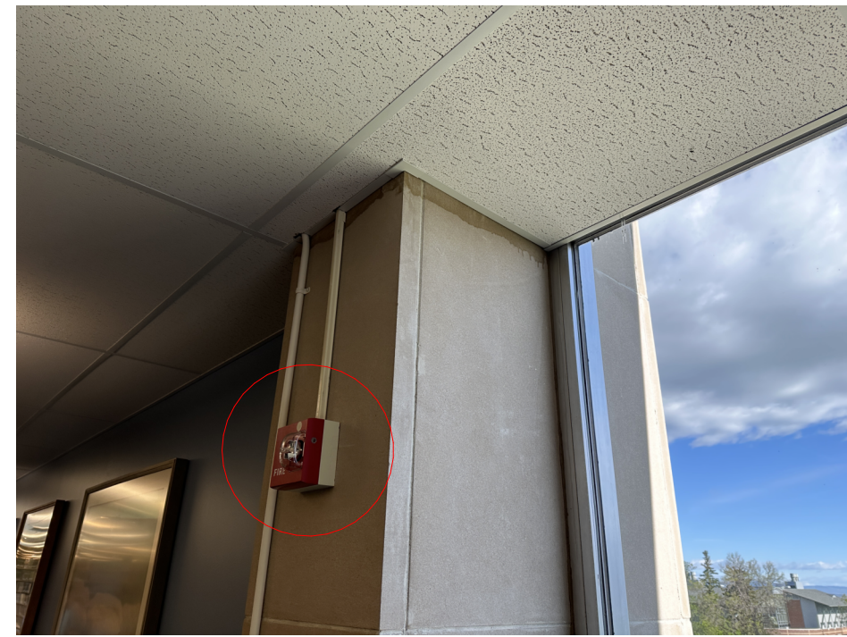
PHOTO OF EXISTING FIRE DEVICE LOCATED AT GRID LINE 4-A TO REMAIN.
