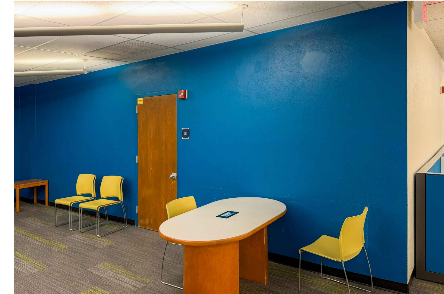
PHOTO 1: REMOVE PLASTER WALL SYSTEM AND UNDERLYING RACM BONDING AGENT COMPLETELY FROM THE WALL ALONG THE SOUTH SIDE OF ROOM 216ME (PAINTED BLUE IN PHOTO). SEE DETAIL NOTES.
