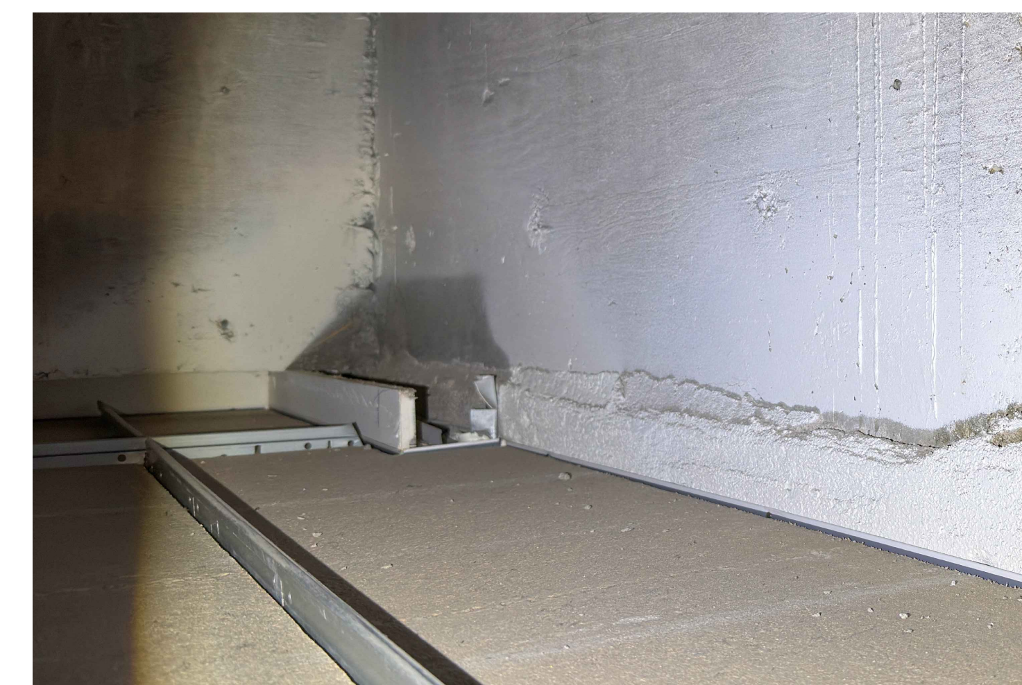
PHOTO 3: PLASTER WALL SYSTEM ON CONCRETE WALL SUBSTRATE. VIEW IS ABOVE THE EXISTING LEARNING STUDIO LAY-IN CEILING, LOOKING TOWARD THE WEST END OF THE WALL ALONG THE SOUTH SIDE OF ROOM 216ME. PLASTER EXTENDS APPROXIMATELY 4 TO 6 INCHES ABOVE THE CEILING GRID.
