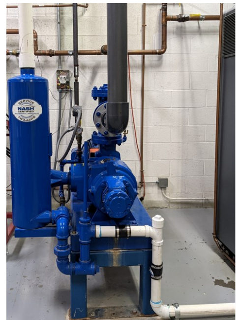
Liquid ring vacuum pumps for line 4
