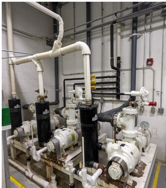
Liquid ring vacuum pumps for lines 1, 2 and 3
